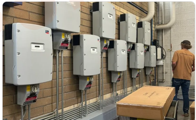
Inverter tested under load; age and fault history recorded
